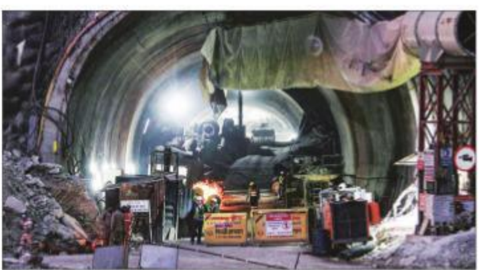
NDRF personnel at the under-construction tunnel between Silkyara and Dandalgaon, days after a portion of the tunnel collapsed trapping several workers inside, in Uttarkashi on Tuesday
